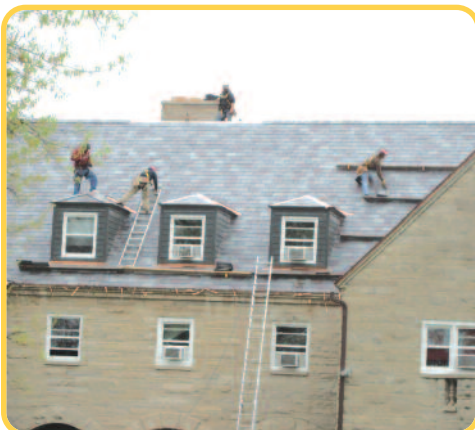
Rain or shine, construction workers were hard at work to replace the slate roof and gutter system.
