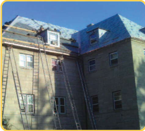
Alumni contributions to the annual fund have made the new roof possible.
